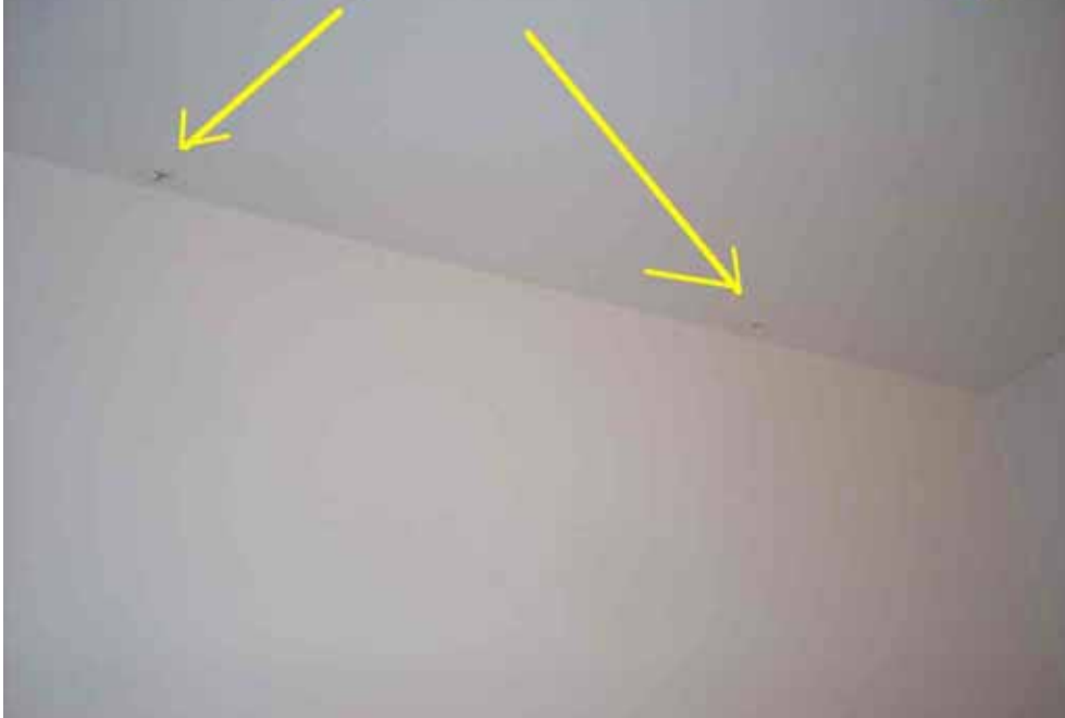
#40 Nail pops in bathroom ceiling.
